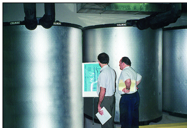
Two 1,600-gal. Ice Storage Tanks
