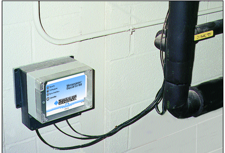
Triangular Wave System (coil hidden by insulation)
